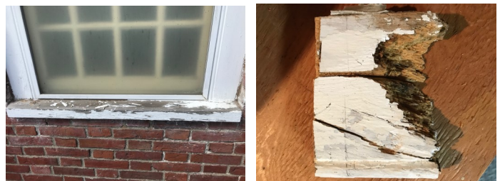
Left: Windowsill before painting; Right: rotted wood
